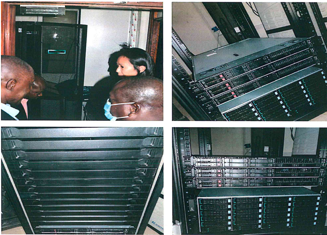
Figure 1: Showing servers at LGFC
