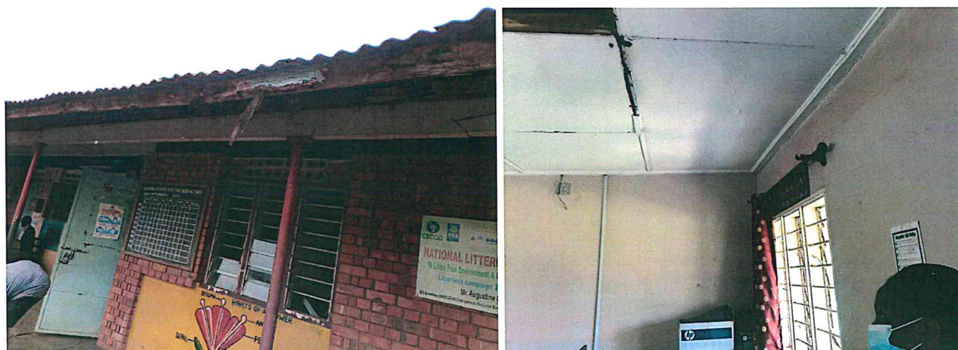
Figure 21&22: Showing Administrative block for Ntinda school for the deaf before renovation
