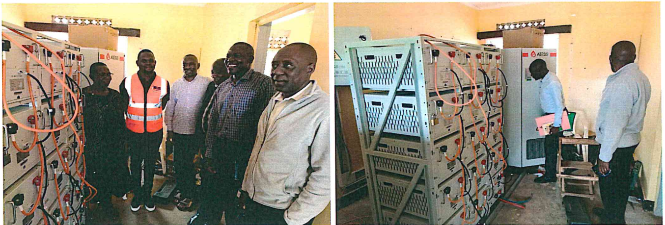
Figure 36&37 Power room for the three Phase Hybrid solar system installed at Ntinda School for the deaf.
