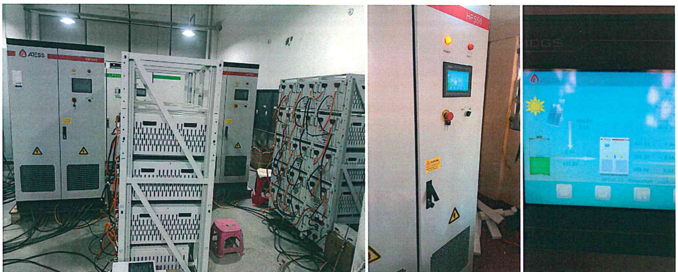
Figure 32 &33 showing Power room for the three Phase Hybrid solar system installed at Mulago School for the deaf
