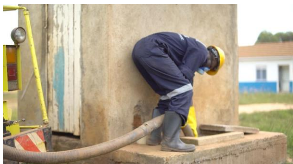
Figure 6: Safe Emptying of a lined toilet
